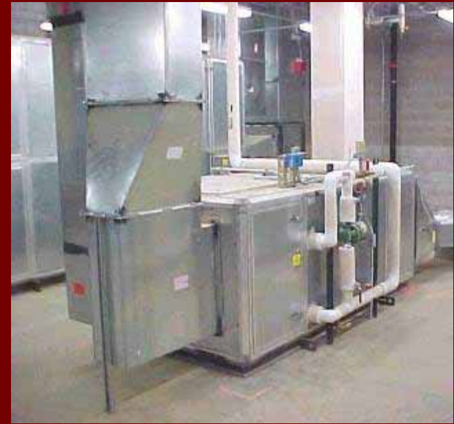
HVAC, power meters
